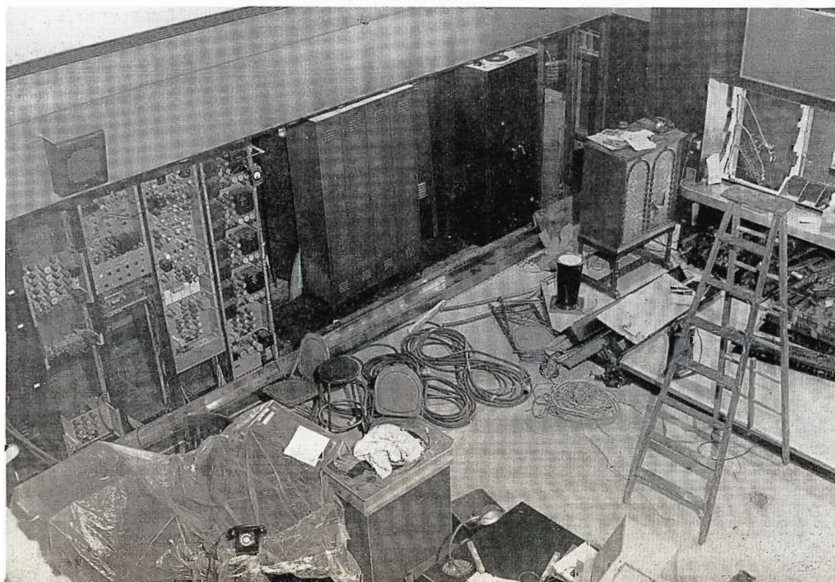
FIG. 5 (bottom). And this is how "old master" looked in January, in the midst of the conversion which will make it the "Video Central" of WNBQ's all-color operation. Radio operations have been transferred to a new radio control room in the front section of the building. All of the audio racks have been pulled out, and the big control board (top right) is on the way to the junk yard. In the new setup all color video control positions and associated equipment for live and film cameras will be located in this room. Video racks will line the room (where audio once stood). Camera control units will form a console in the center. One live color camera chain is already in position (racks at left center, camera control under the plastic covering).
