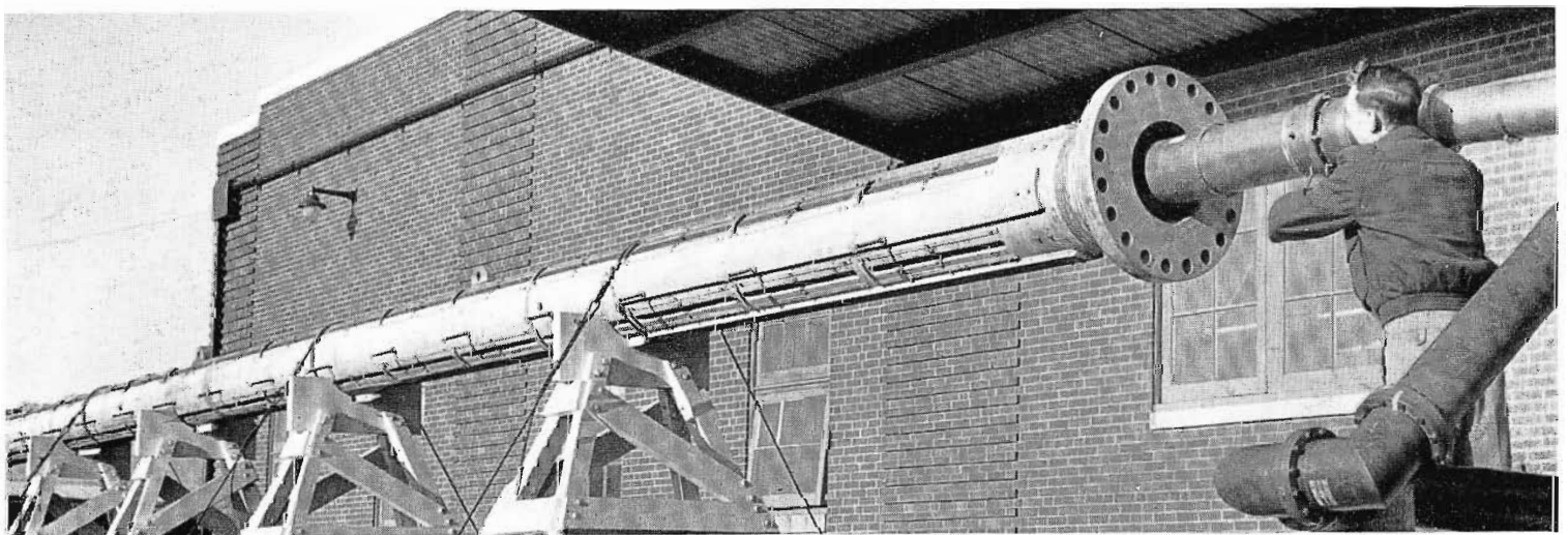
Approximately 4½ megawatts are produced by feeding 100 kilowatts into this super-power antenna with a gain of nearly 50.
