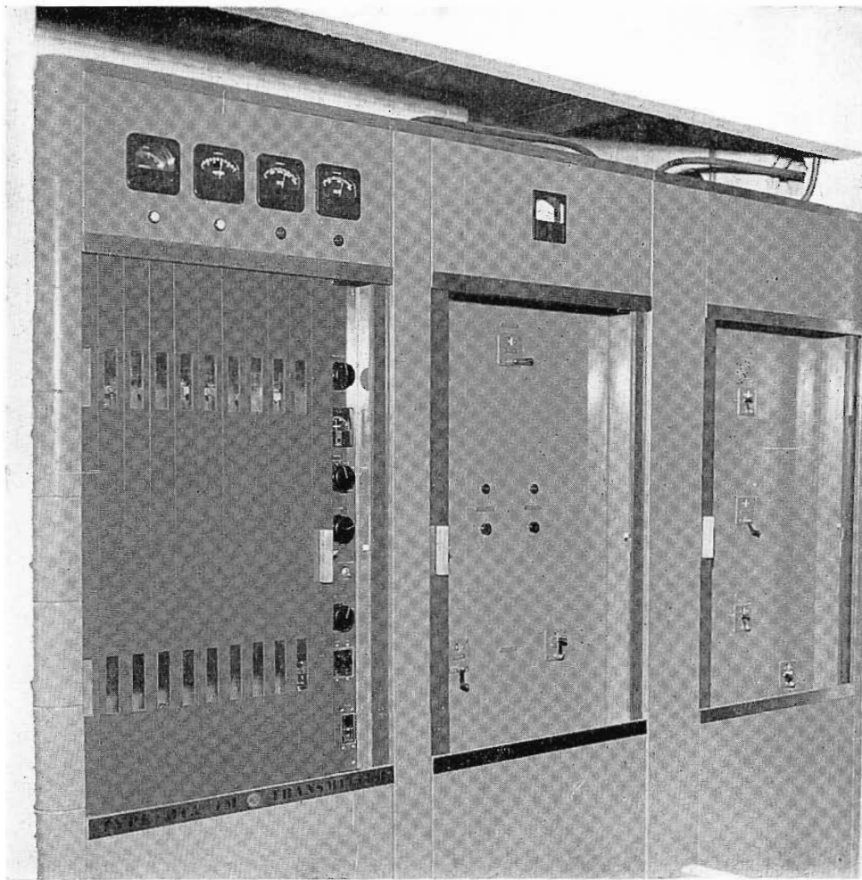
FIG. 4. RCA BTA-1M 1 kilowatt transmitter, left, with power dividing and branching equipment mounted in two matching right wing phasing cabinets. Day/night switching facilities are in cabinet directly to right of BTA-1M.
